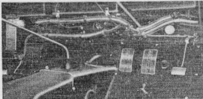
Fig.46. General view of Heater Water Pipes.
